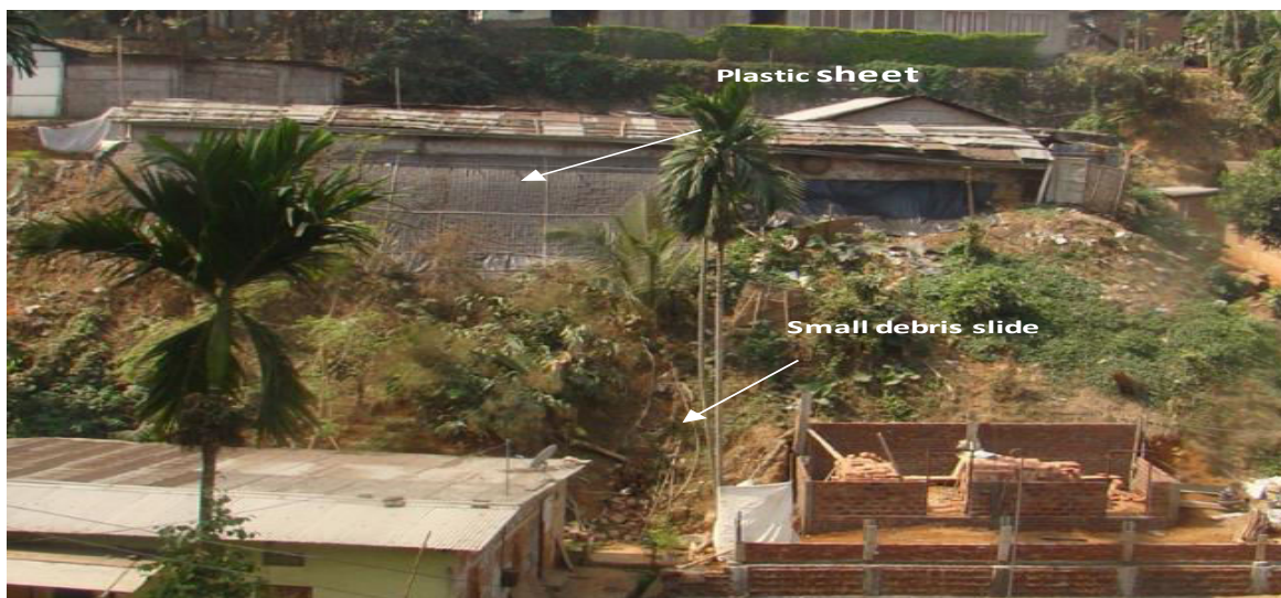
Fig.7: Field photographs from Guwahati city, Assam. Plastic sheet is spread to arrest rainfall percolating the slope. Source: NESAC/ATLAS/01/2013.
